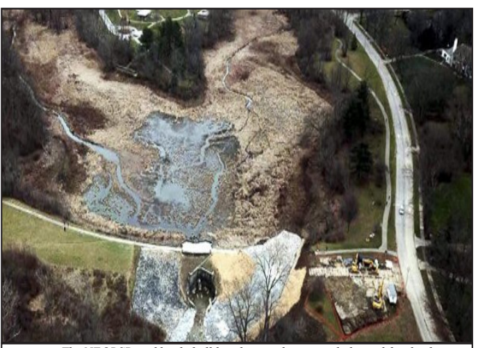
The NEORSRD recklessly bulldozed, tagged trees, and planned for the destruction of the historic Horseshoe Lake. The utility ignored the areas historic federal protections. The utility neglected to inform residents of the $200 M Doan Valley tunnel which they had dug at the bottom of Ambler Park to prevent flooding in University Circle. Most distressing to the residents was the NEORSRD's complete lack of concern for the wildlife as the NEORSRD allowed fish, frogs, snails and turtles to die. A lawsuit is currently in federal court to stop the NEORSRD's plan. Please send a comment (left) to support the Shaker Lakes.
